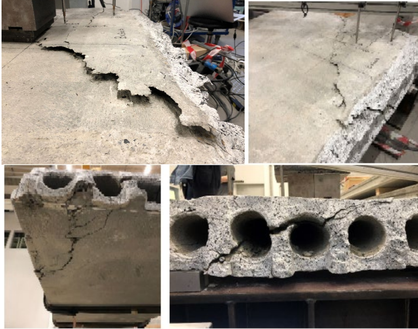
Fig. 6. Pictures of Specimen R-2.b after failure; (top, left and right) failure seen from the upside of the slab, (bottom, left) failure seen from the bottom of the slab and (bottom, right) failure seen from the end of the slab.
